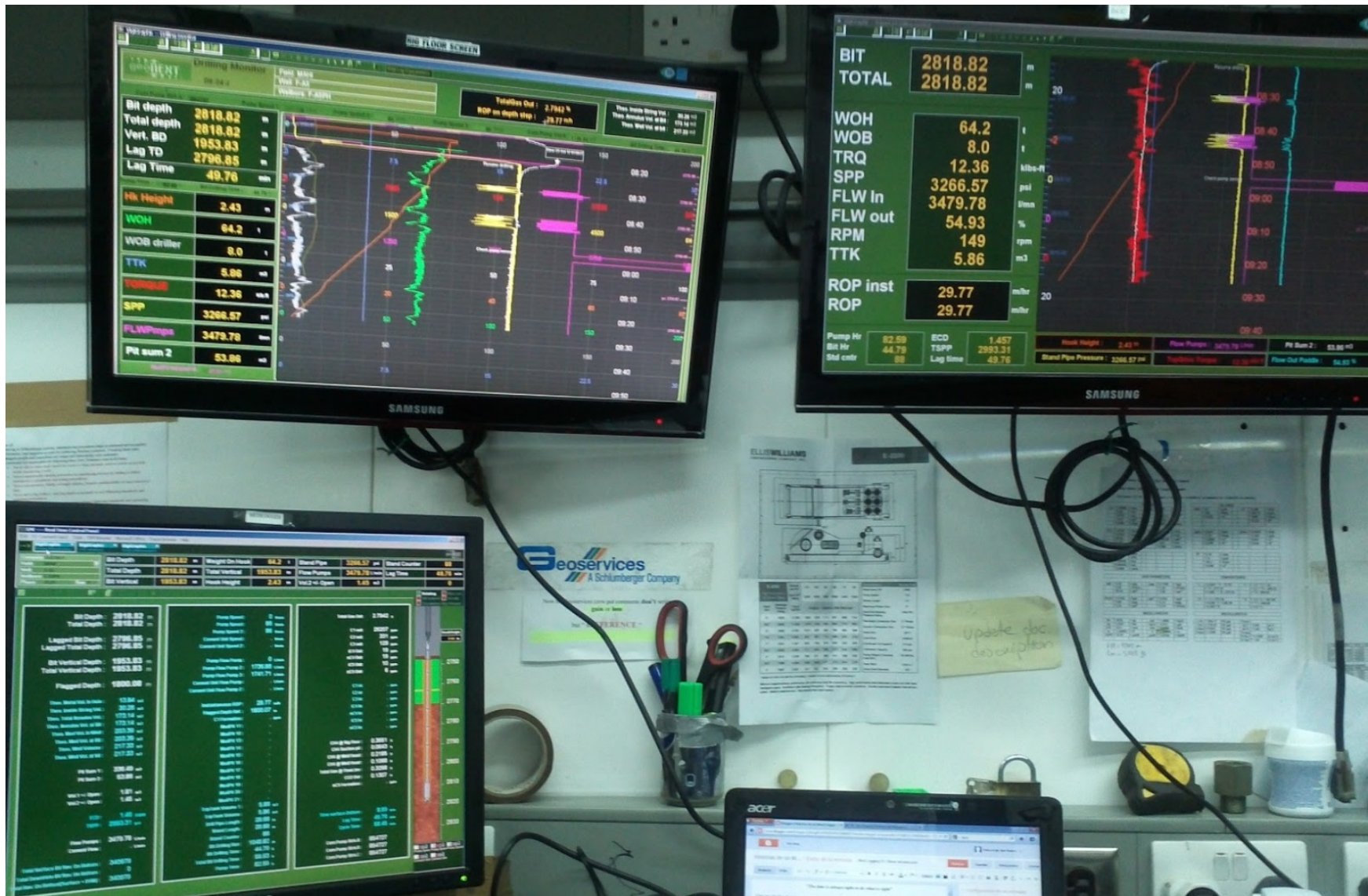
Figure 5.9: Real-time drilling monitoring equipment.
