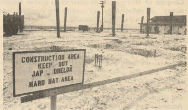
A new hospital is under construction on Ebeye, home of more than 5,000 Marshallese many of whom work at Kwajalein. But the project has been delayed, mostly by supply shipping problems. The hospital should be completed by early next year, says Ebeye DistAd Rep Murph Ownby.
