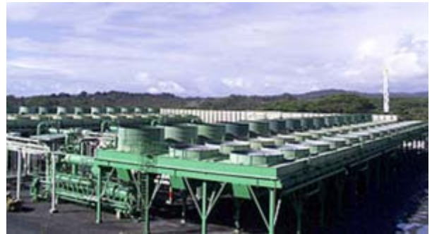
Fig. 1: Puna Geothermal Venture (PGV) power plant. (Courtesy of the DOE )
