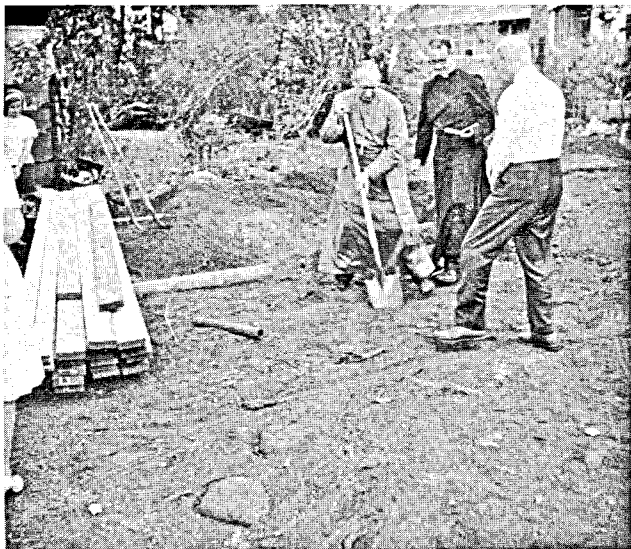
Groundbreaking for the new classroom building at Church of the Good Shepherd, Wailuku, Maui. The Reverend Roger M. Melrose, and Mr. Ernest Halford, Senior Warden, watch the Bishop turn the first spade of dirt.
