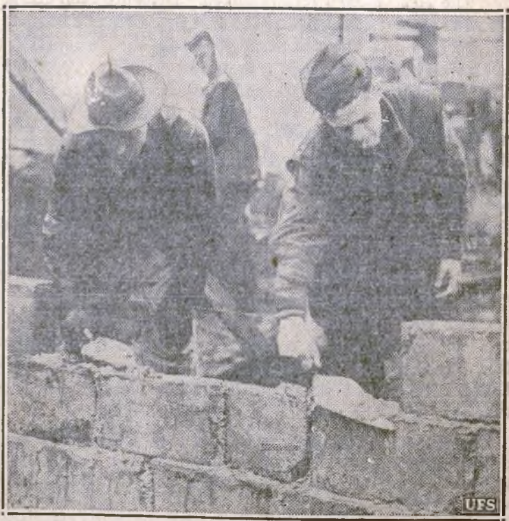
FRATERNAL CEMENT—American Marine and British soldier spread what might be cement of brotherly love, as side by side they build foundation for one of huts that house American troops in Iceland, not long before troops' arrival.
