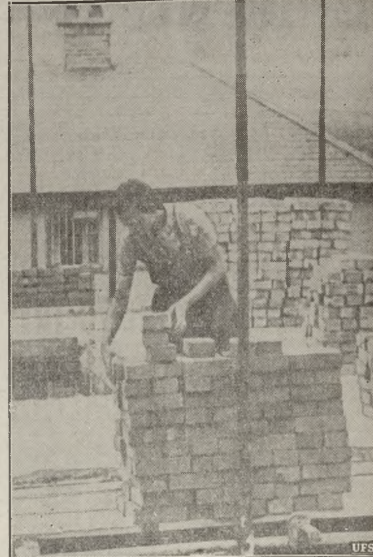
WOMEN BUILDERS —With men called into service in Britain, women and girls are taking their places in industry. Here's a girl bricklayer at work, helping to build homes for arms workers erected in various parts of Island under direction of British Ministry of Supply.
