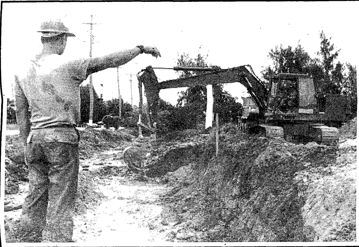
Work goes on by the Naval Mobile Construction Battalion at American Memorial park on Saipan.
